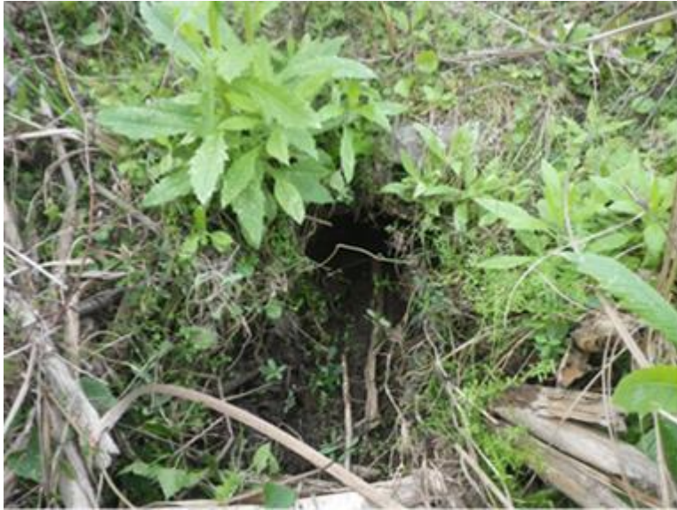
Figure 8. Outlet Location of Occluded Stormwater Culvert
