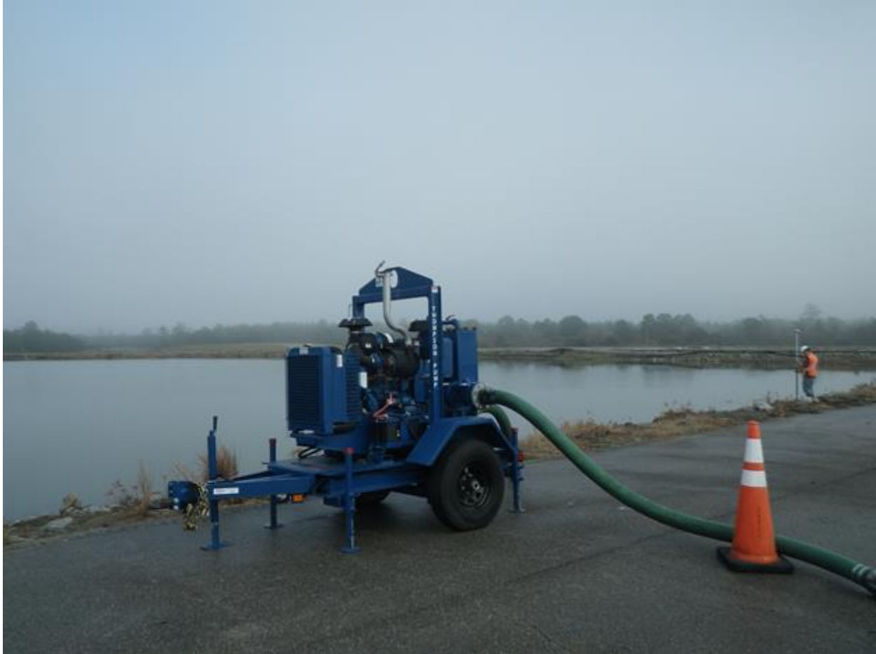
Figure 5. Mobile Pump Transporting Decant Water from Ash Cell #1 to Pump Back Cell #1
