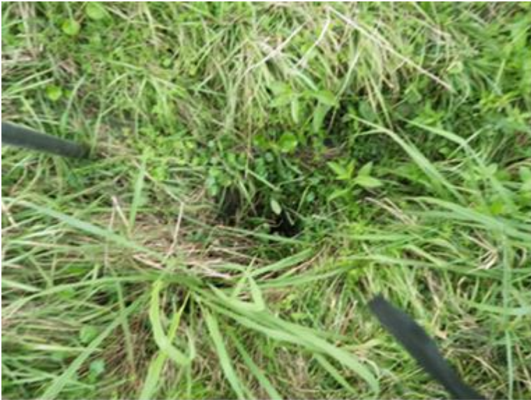
Figure 7. Inlet Location of Occluded Stormwater Culvert
