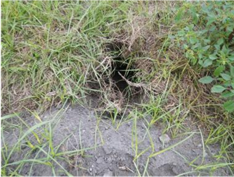
Figure 6. Animal Burrow Located on Landfill Southern Exterior Side Slope
